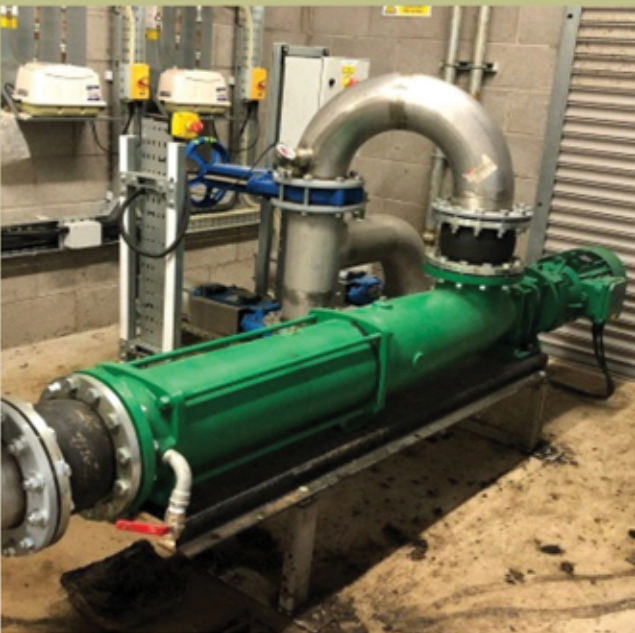
BIOMASS RECIRCULATION PUMP Flow – 80 m 3 /hr, Pressure – 4 bar
