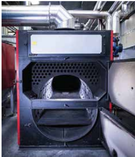
SASP System 1 MW
